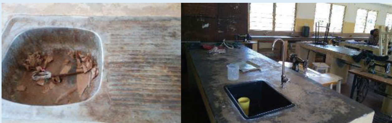
Picture 9: Condition of Laboratories
