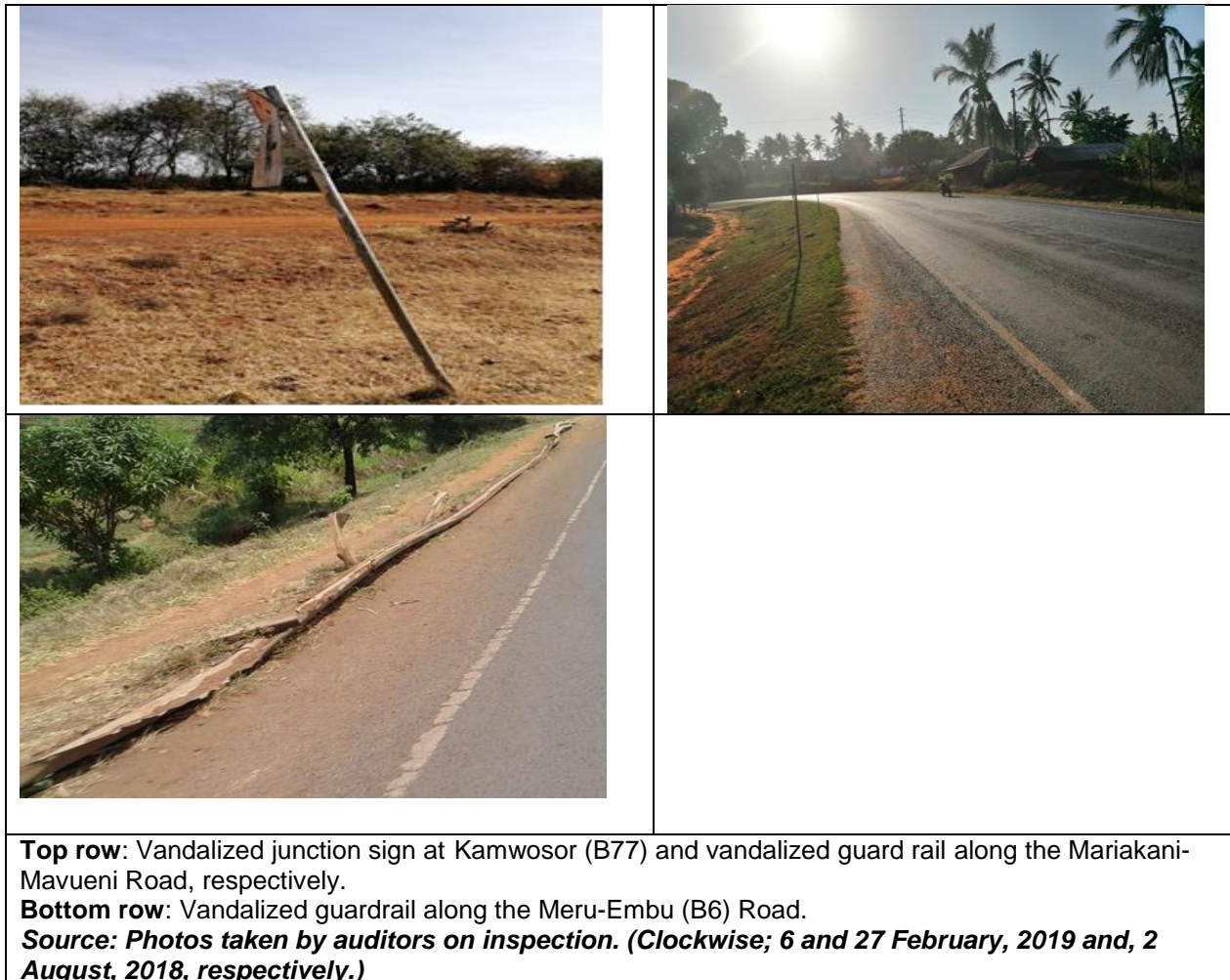
Figure 3: Vandalised Road Furniture
