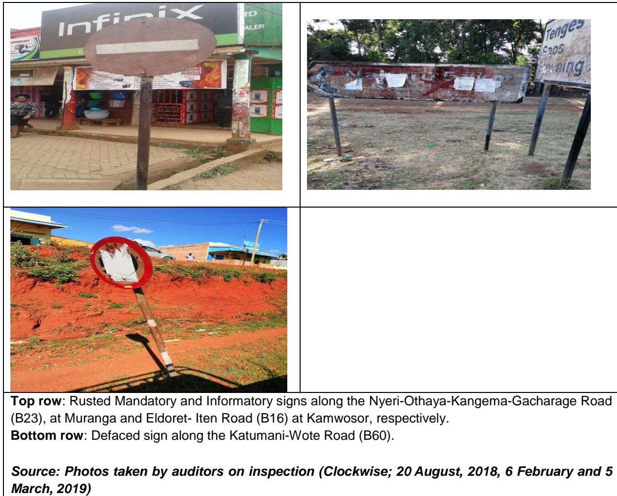
Figure 2: Road Signs that were Defaced, Faded and had Rust
