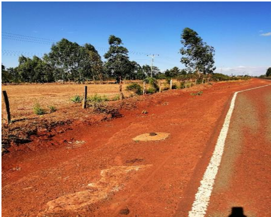
Figure 8: Vandalised Road Furniture
