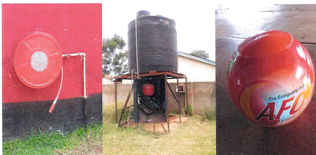
Source: Physical verification of firefighting equipment by OAG Staff
