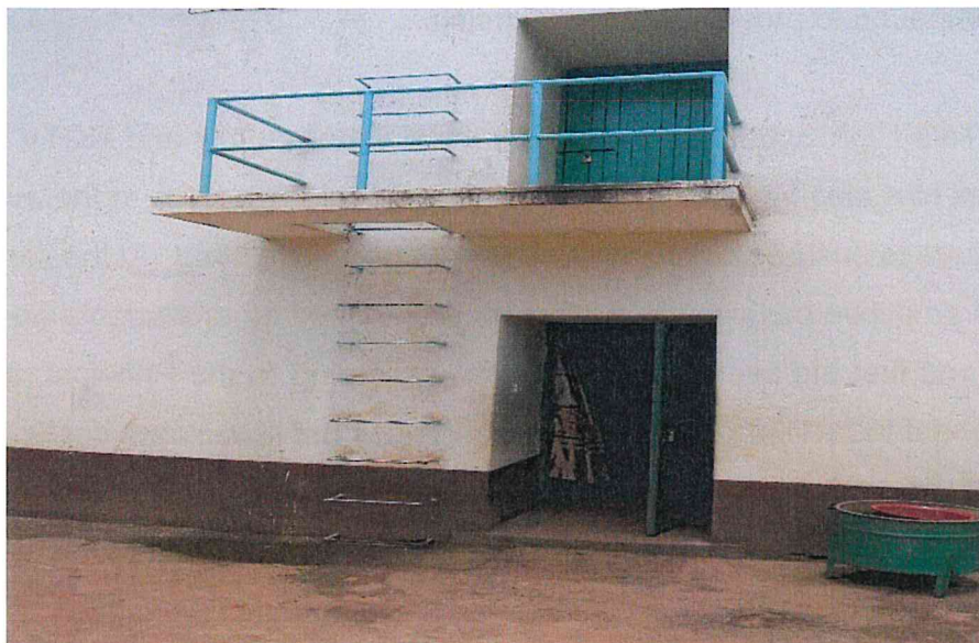
Source: Physical verification of firefighting equipment by OAG Staff
