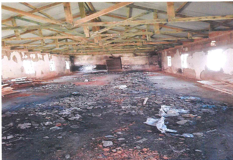
Source: OAG Staff physical verification of school buildings destroyed by fire
