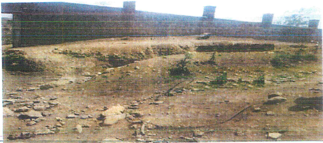
Picture 1: Athi River -Namanga damaged NOFBI phase I section that was not commissioned Source: OAG
