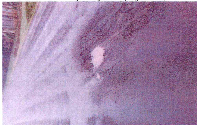
Picture 5: Potholes-Othaya-Konyu Road (August 2014)
