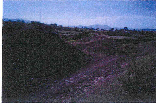
Picture 1: Incomplete sections of Homa-Mbita road (August 2014)
