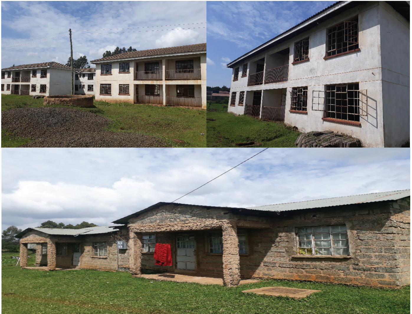
*Top two photos: Stalled Moody Awori houses at about 90% of completion. Bottom photo: Due to housing deficit, officers live in the incomplete RRI houses.
