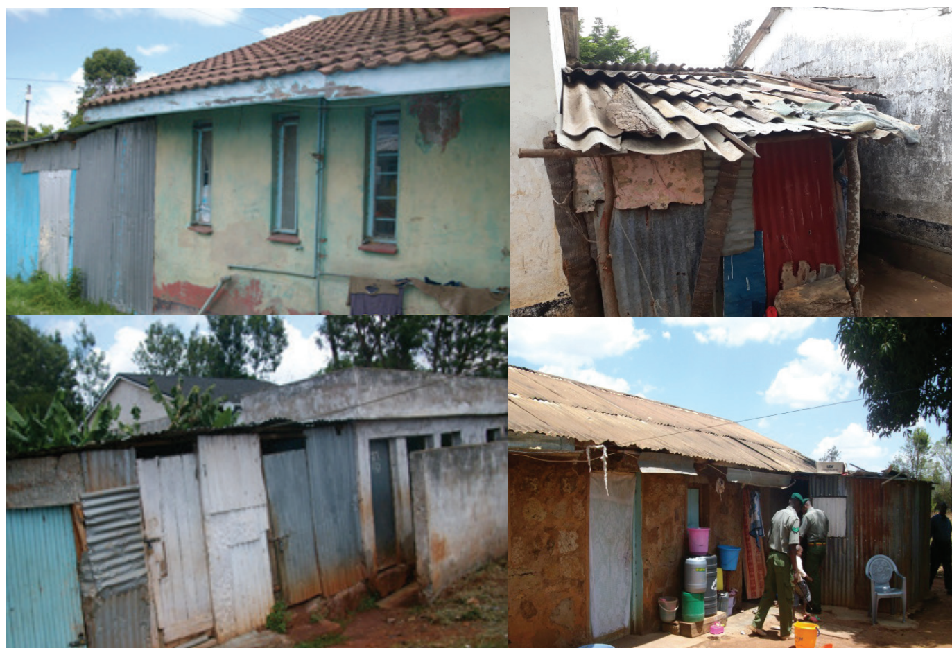
*To address the shortage of houses, officers do extensions and erect uncontrolled structures to create more space.
