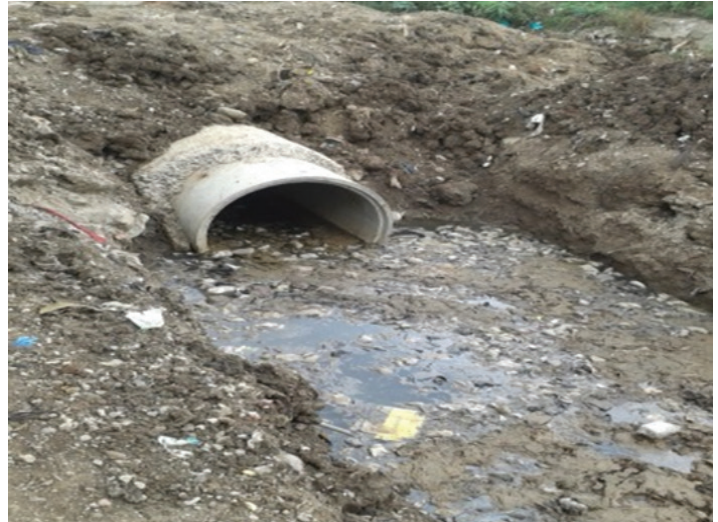
Plate 2: Incomplete section of Sewer Blue Estate, Nairobi
