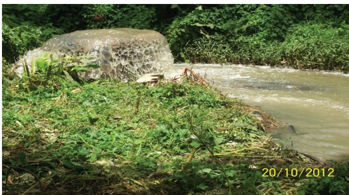
Notice the raw sewage flowing from the manhole causing pollution to Nairobi River
