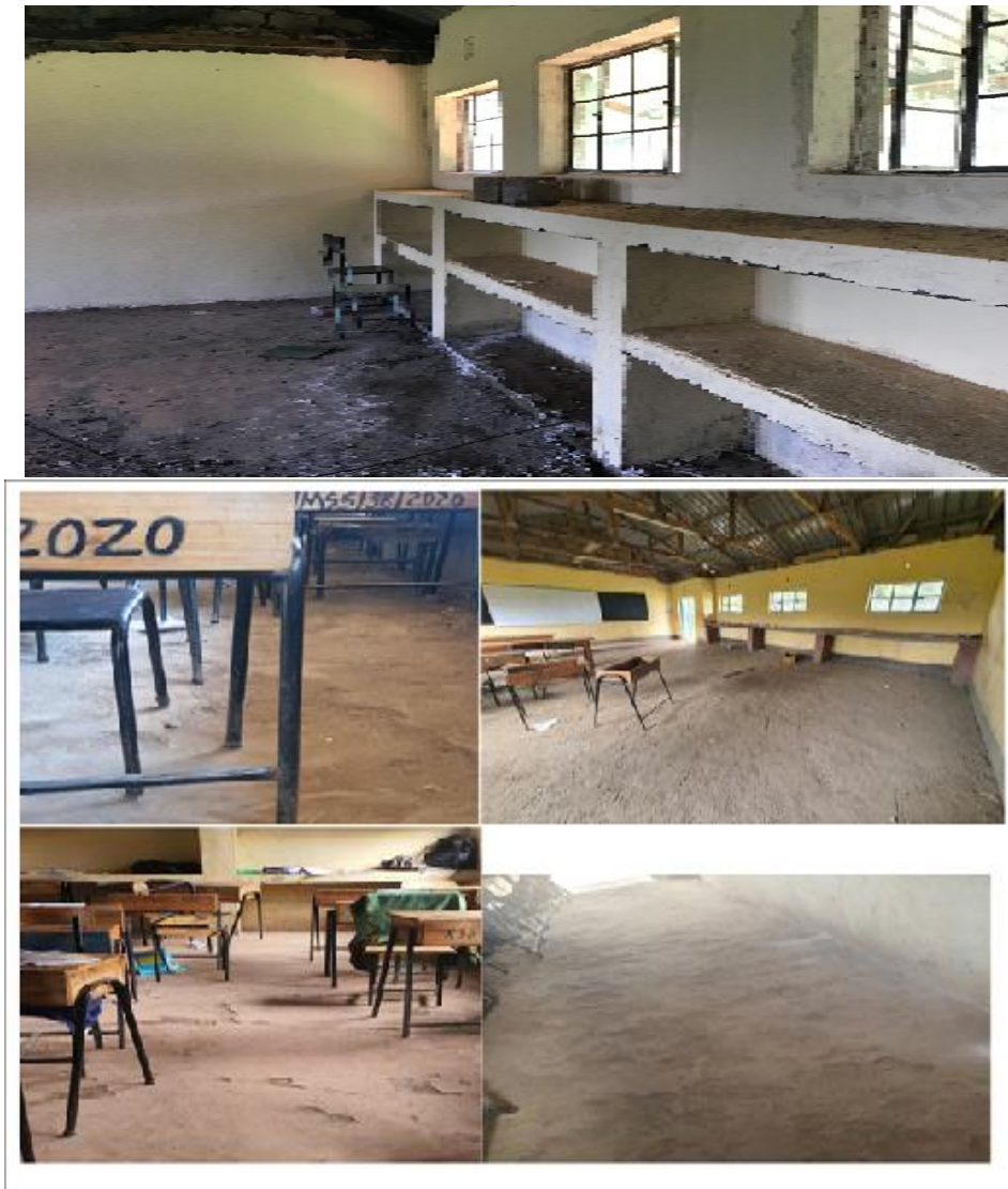
Picture 4: Classrooms with Poorly Constructed Floors
