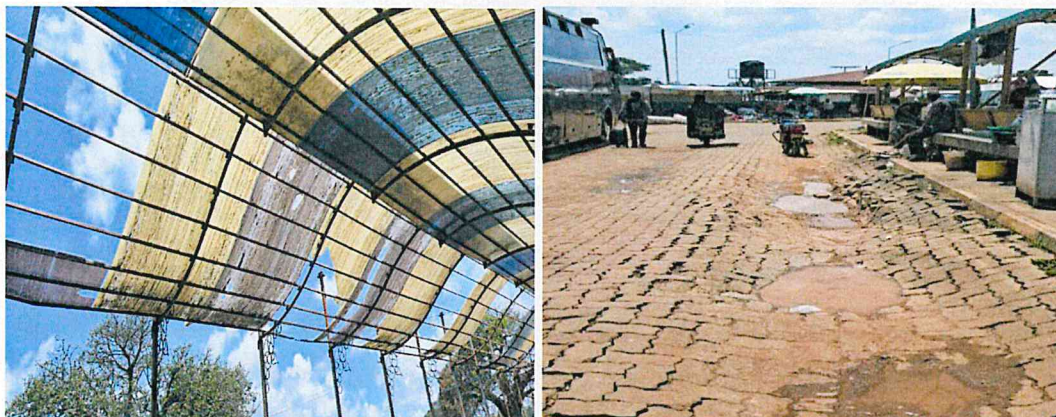
Worn out Roof in Barani NMT project in Malindi and Cabros installed in Mumias Bus Park that need maintenance.
