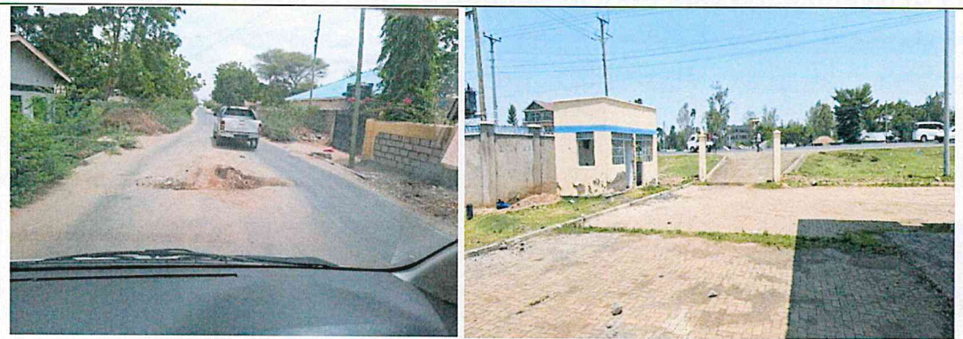
Deep pothole at Galbet Township Road in Garissa and Vandalized Nyamasaria Bus Park in Kisumu whose security office has no doors and windows.
